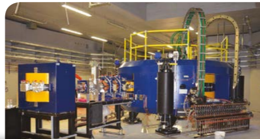
Installation of Best 70 MeV Cyclotron at Italian National Laboratories (INFN), Legnaro, IT
